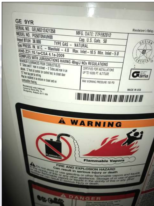
Hot water heater nine years old
